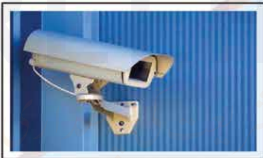
CCTV Camera 24 hours Services
